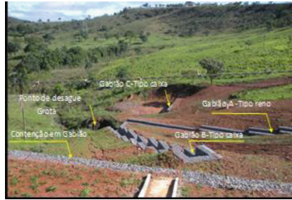
Fig. 27. System implanted with the completion of the work.
