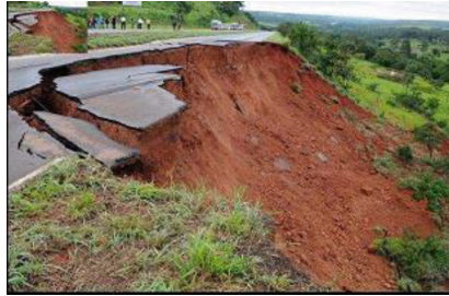
Fig. 3. Broken section of the BR-060/GO (12/31/2010).
