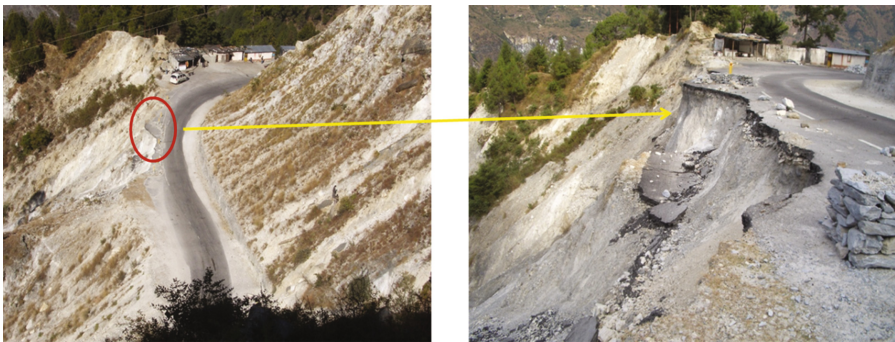
Fig. 3. Highway at risk due to debris slide
