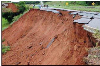
Fig. 4. Broken section of the BR-060/GO (12/31/2010).
