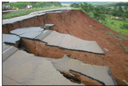
Fig. 5. Broken section of the BR-060/GO (12/31/2010).
